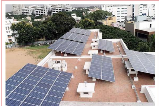
Installed Solar Panels at Surangi Unit, reducing 80 MT carbon emissions per month
